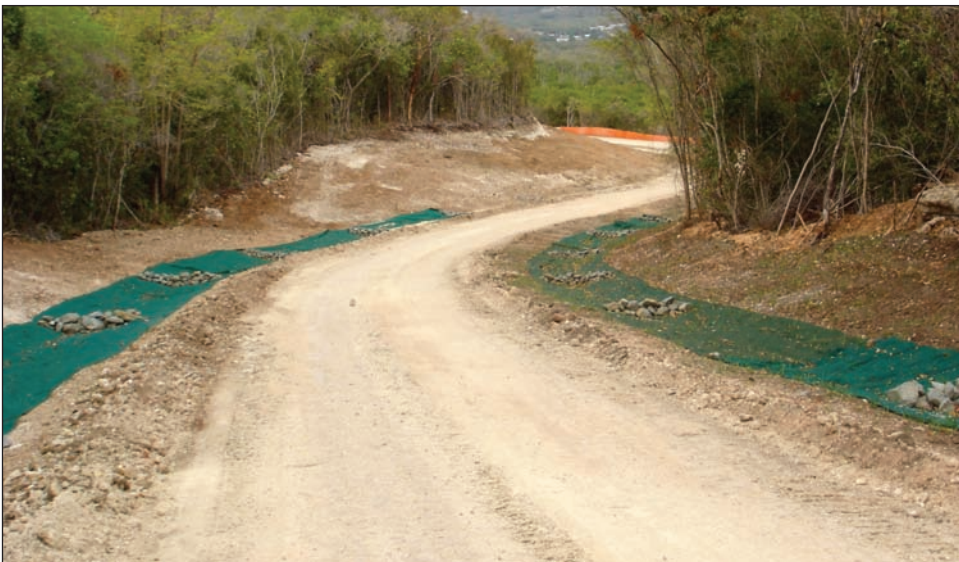
Fig. 49. The Puerto Ferro replacement road in 2008 destroyed native habitat for flora and fauna of conservation concern. The large shoulder areas are now covered by nonnative thorn scrub. (Puerto Ferro Replacement Road, Gemmill 2008)
